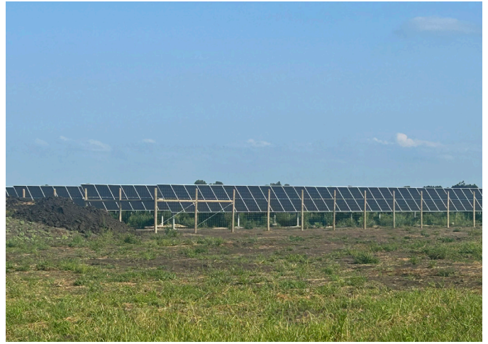
Ground-Mounted Solar Panels in Lisbon
