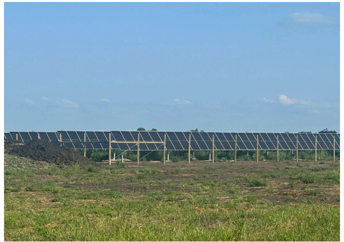
Ground-Mounted Solar Panels in Lisbon
